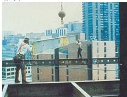
At-risk workers without appropriate safety equipment
